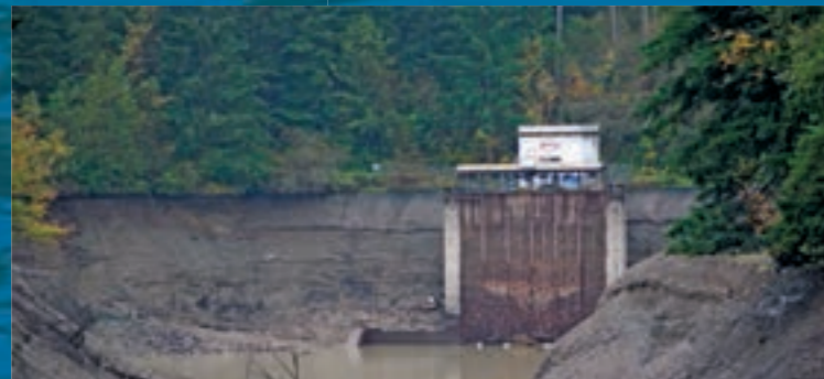
Lower Conveyance Assessment and Trash Rack Intake Inspect intake tunnel, forebay and penstocks; replace intake trash rack and stop logs; decommission Penstock No. 4; conduct additional repairs as necessary
