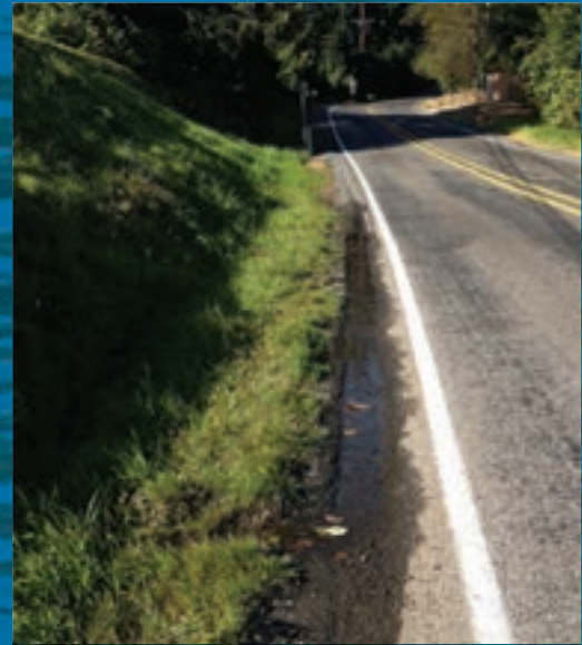
Dike 3 Seismic Remediation To make the dike earthquake safe, and work to stop water seepage
