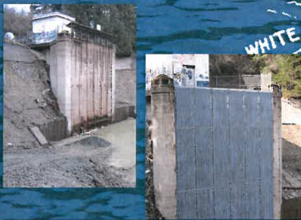
Lower Conveyor Assessment and Tunnel Intake Inspected intake tunnel, forebay and penstocks; replaced intake trash rack with new steel 45 feet across and 53 feet high and made new stop logs; decommissioned Penstock No. 4.
