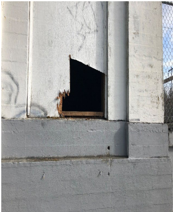
1. Vandalism - ½ mile above Powerhouse.
