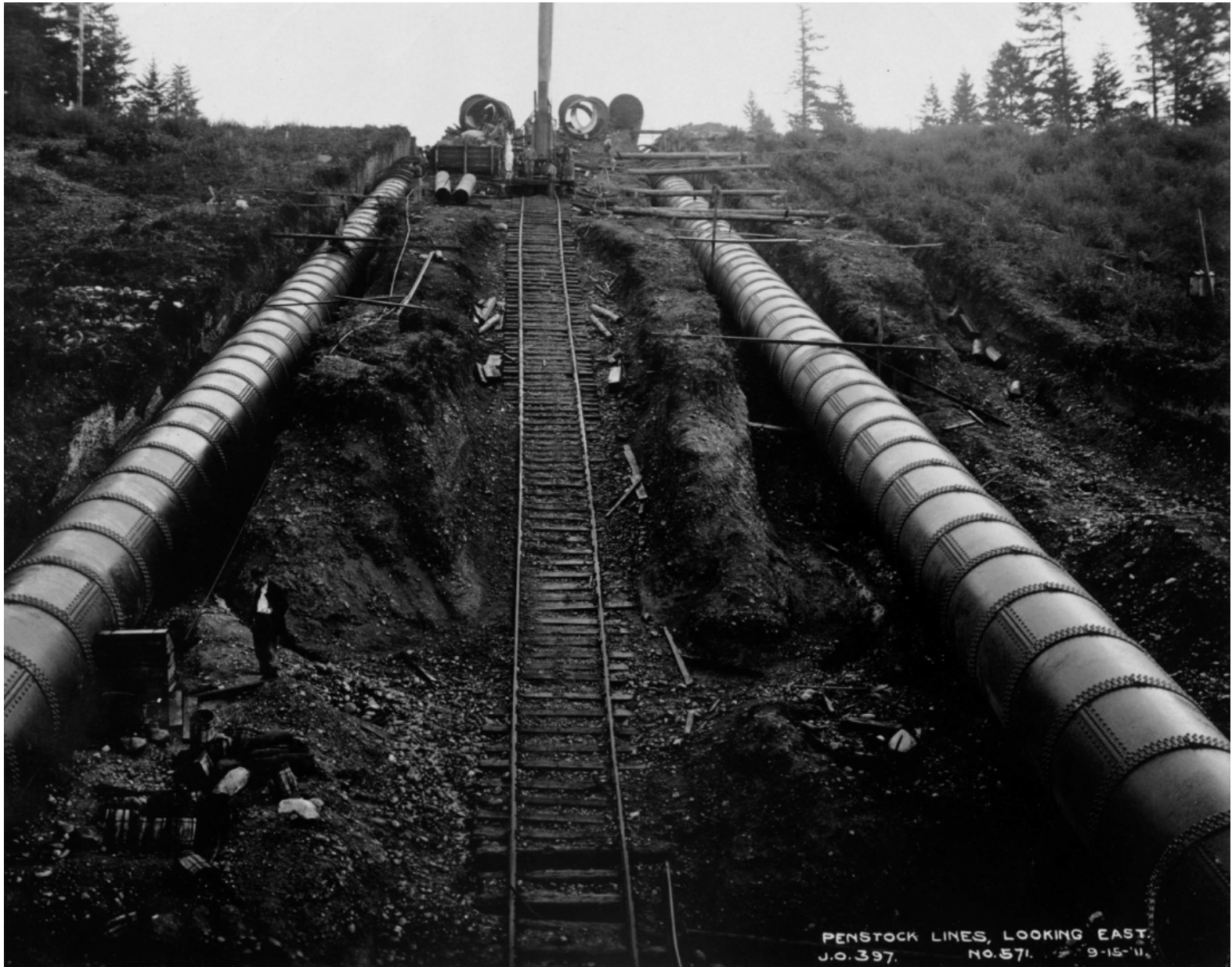
Penstocks 1 (left) and 2 (right). Railroad track and boom in middle to set pipe. 9-15-11
