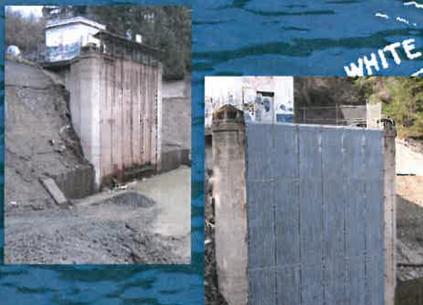
Lower Conveyor Assessment and Tunnel Intake Inspected intake tunnel, forebay and penstocks; replaced intake trash rack with new steel 45 feet across and 53 feet high and made new stop logs; decommissioned Penstock No. 4.
