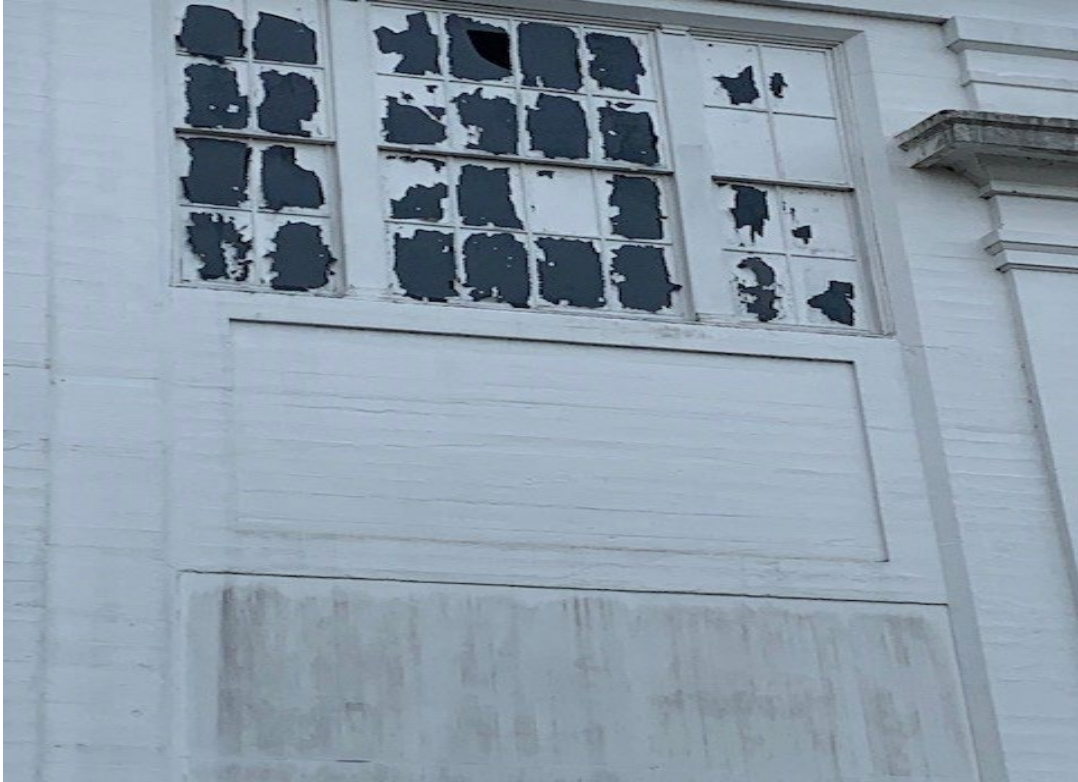
Old Windows Needing Replacement at the Powerhouse
