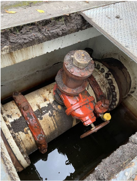
Bellevue-Issaquah Pipeline “pig station”
