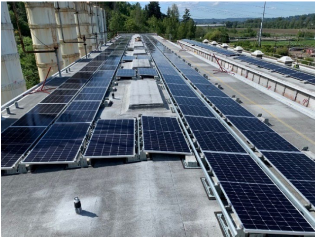
Solar panels installed on the Powerhouse in 2022.
