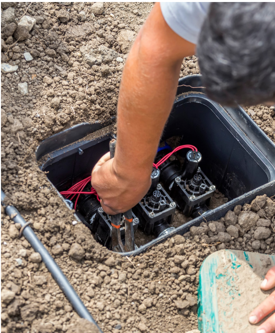
An irrigation valve box
